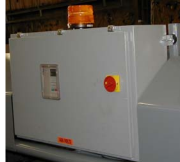
Control Cabinet with drive window.
